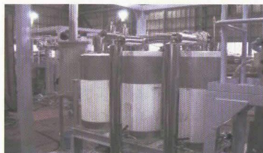
Fig.6 Detail view of reactors
