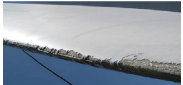
Fig.3 Rotor blade leading edge erosion. 1)
