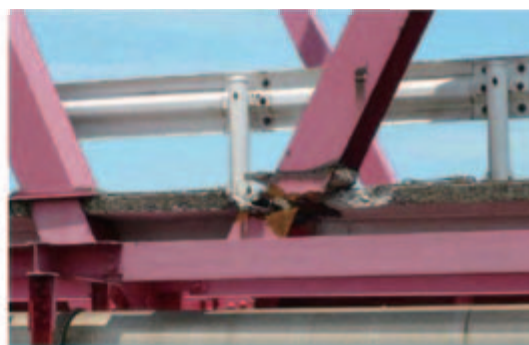
Failure of Kisogawa river truss bridge http://www.tohokukk.jp/by Y. Takeuchi
