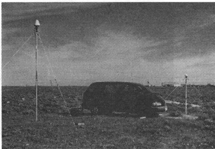
Fig. 8 DGPS Ground Equipment
