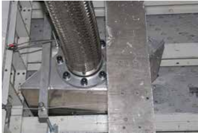
Figure 17: Set up of the can in the plenum.
