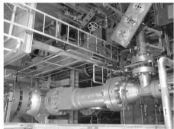
Fig. 2.2.4 A bird-eye's view of the SAH, the hot train, the hot valve and the bypass air mixer from the left.
