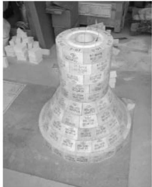
Fig. 5.3 Radiation dome installed in the upper part of the SAH.
