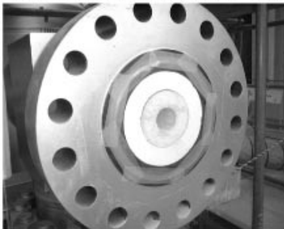
Fig. 5.2 The hot air port from the storage heater connected to the hot valve.
