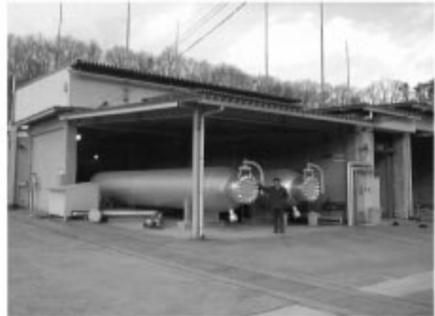
Fig. 2.1.1 The two air storage tanks in the RJTF ( 23\text{MPa} ; 13\text{m}^3 \times 2 tanks).
