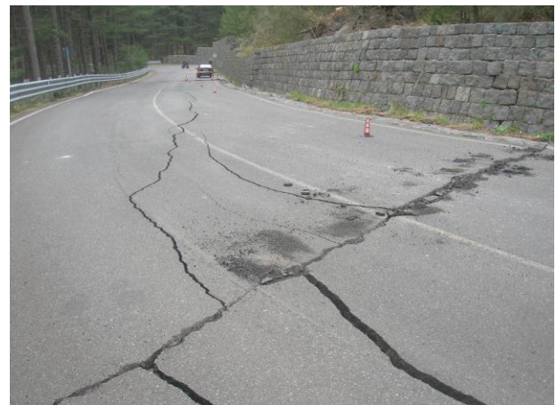
Fig 10. Surface ruptures along the Pernicana fault
